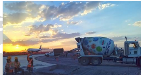
International Airport Felipe Angeles in Santa Lucía
