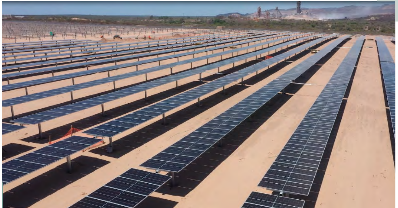
■ Solar park in San Luis (Argentina)
