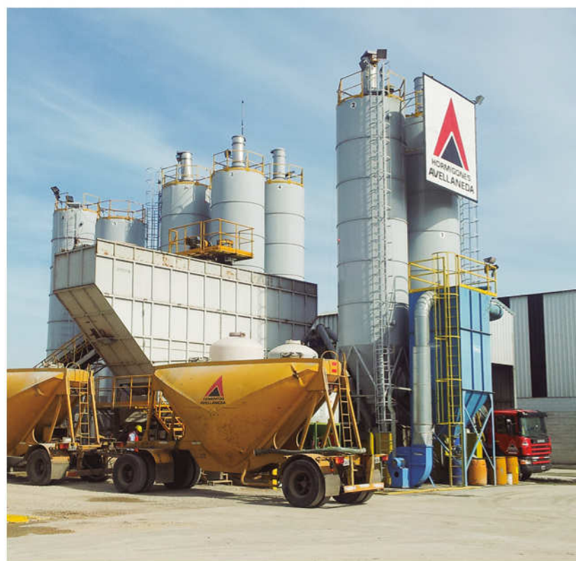
> Concrete production facilities. Argentina.
